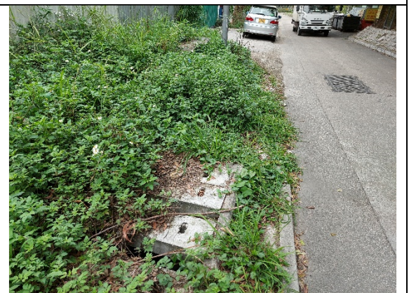
Plate No. 6 – Existing Catchpit 2 which should receive flow from an existing 450U channel and discharge into an existing 525mm diameter drain with respect to the GEOINFO Map
