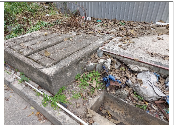
Plate No. 4 – Existing Catchpit 1 and the adjacent existing U channel which is separated from the Existing Catchpit 1 and conveys flow toward Castle Peak Road – Hung Shui Kiu
